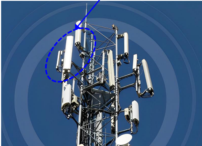
Huawei: Remote Electrical Tilt (RET) antenna [1]
